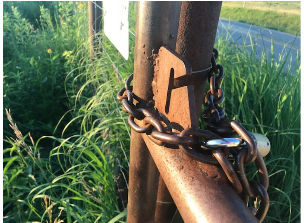
Wrong way to lock gate
